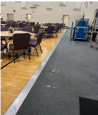
Worn and damaged carpeting around the perimeter of the gym to be replaced with new high quality, LVT flooring
